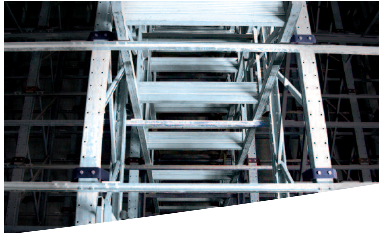
Customer-owned bar stock cradle inside Honeycomb steel structure.
