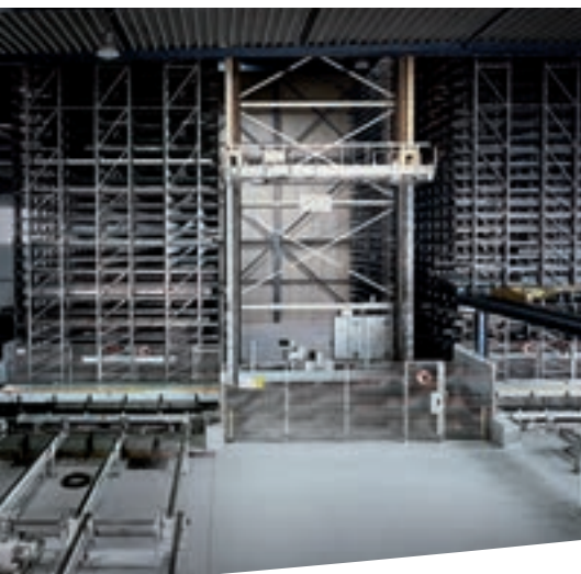
Commissioning storage system for bright steel and non-ferrous metals in service centers.
