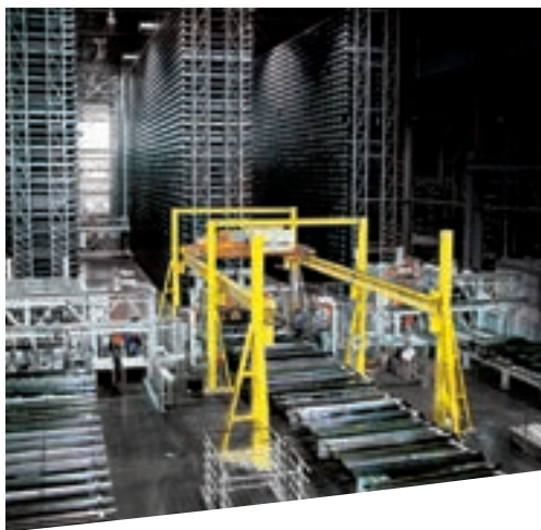
Largest commissioning storage system at a service center in the USA with fully automatic commissioning solution.
