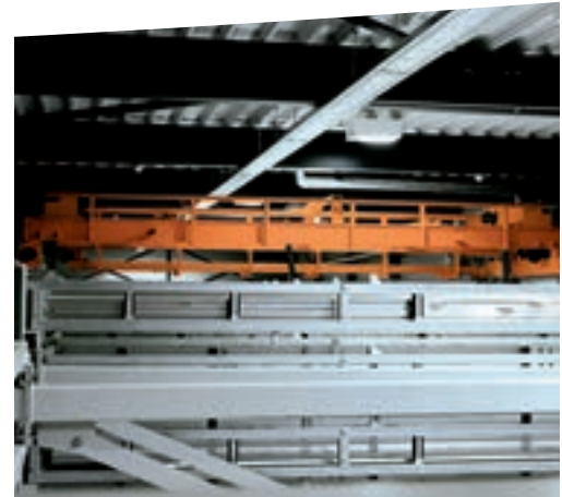
Overhead travel system for racks provided by the customer in window manufacturing.
